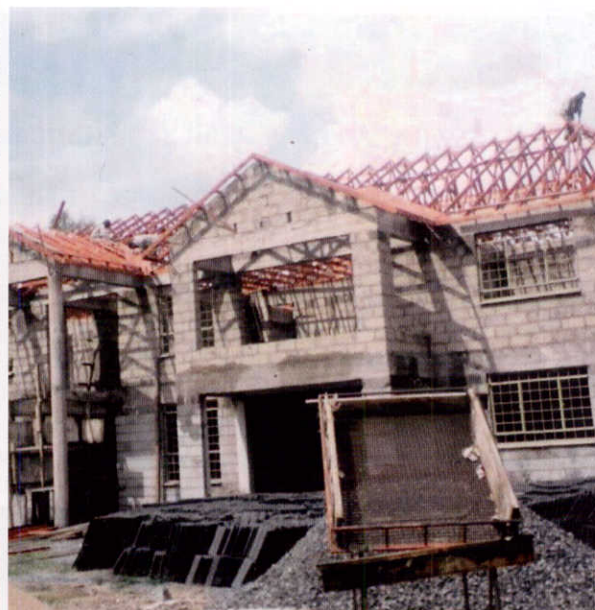
Trussed rafters made from graded cypress timber put into place on residential property in Nairobi. The rafters are designed to carry concrete tiles.
